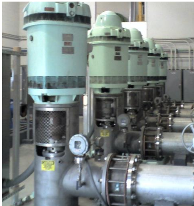
Feed Water Pumps Just After Anti-scalant Injection
