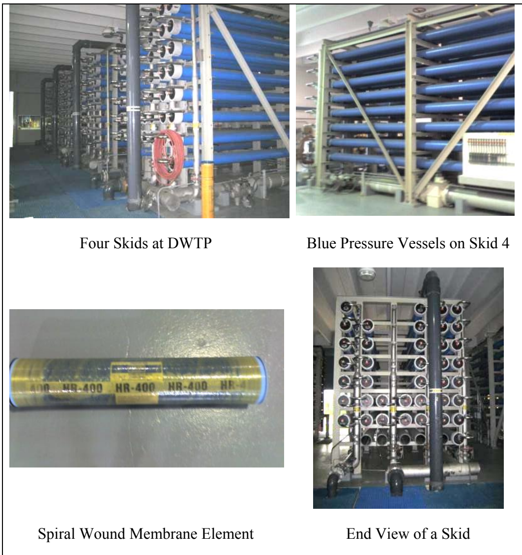
Figure 1: Pictures of RO Skid at the DWTP
